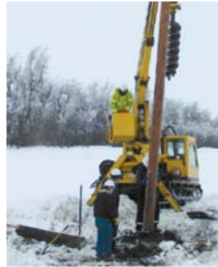
Storm damage costs BHEC thousands of dollars a year, adding to the cost of power.
